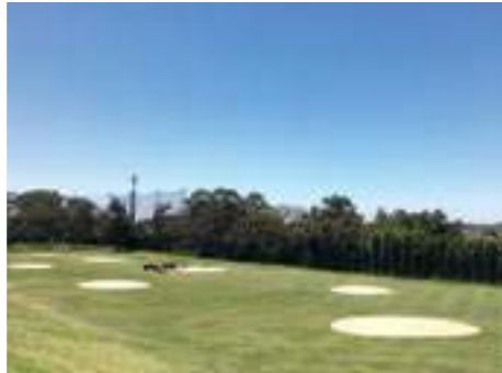
Creating a new 3 rd tee at the 1 st to enlarge tee space.
